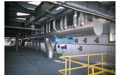
Ammonia Header And Take-Off Trunks
