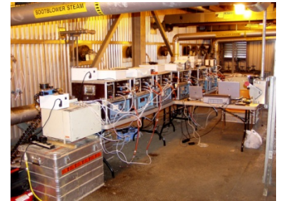
Multi-point NO x /O 2 Analyzer Set-up
